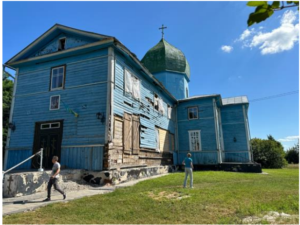
Documenting damage caused by Russian shelling in the village of Peremoha, Kyiv Region. Maidan Museum expedition, August 2023. Photo Khanenko-Friesen.
